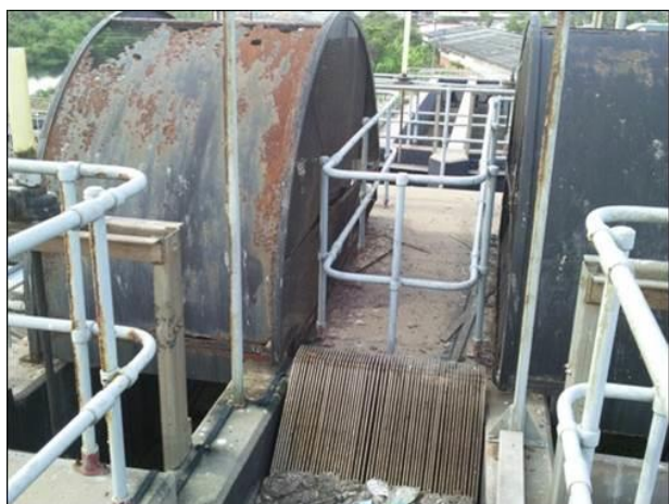
Figure 4.7: Jamestown WWTP - filter shroud rusted through
